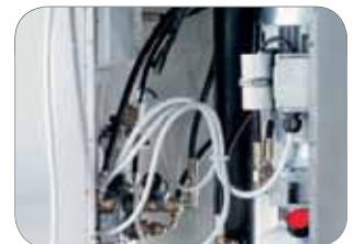
4. Particolare centralina e comandi Electric station and controls
